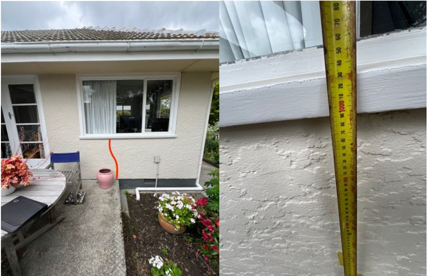
Figure 1 & 2: East elevation (entrance). Signs of cracking in Stucco.
