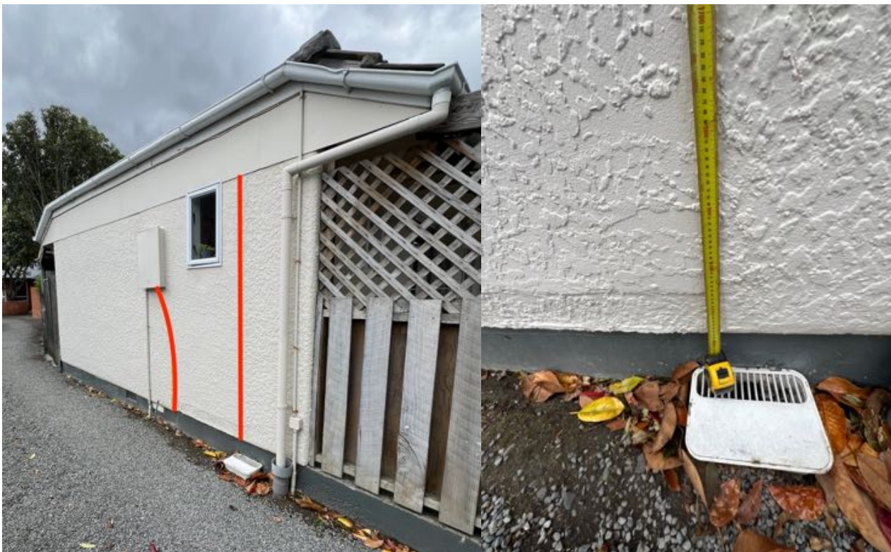
Figure 13 & 14: East elevation (driveway). Signs of cracking in Stucco.
