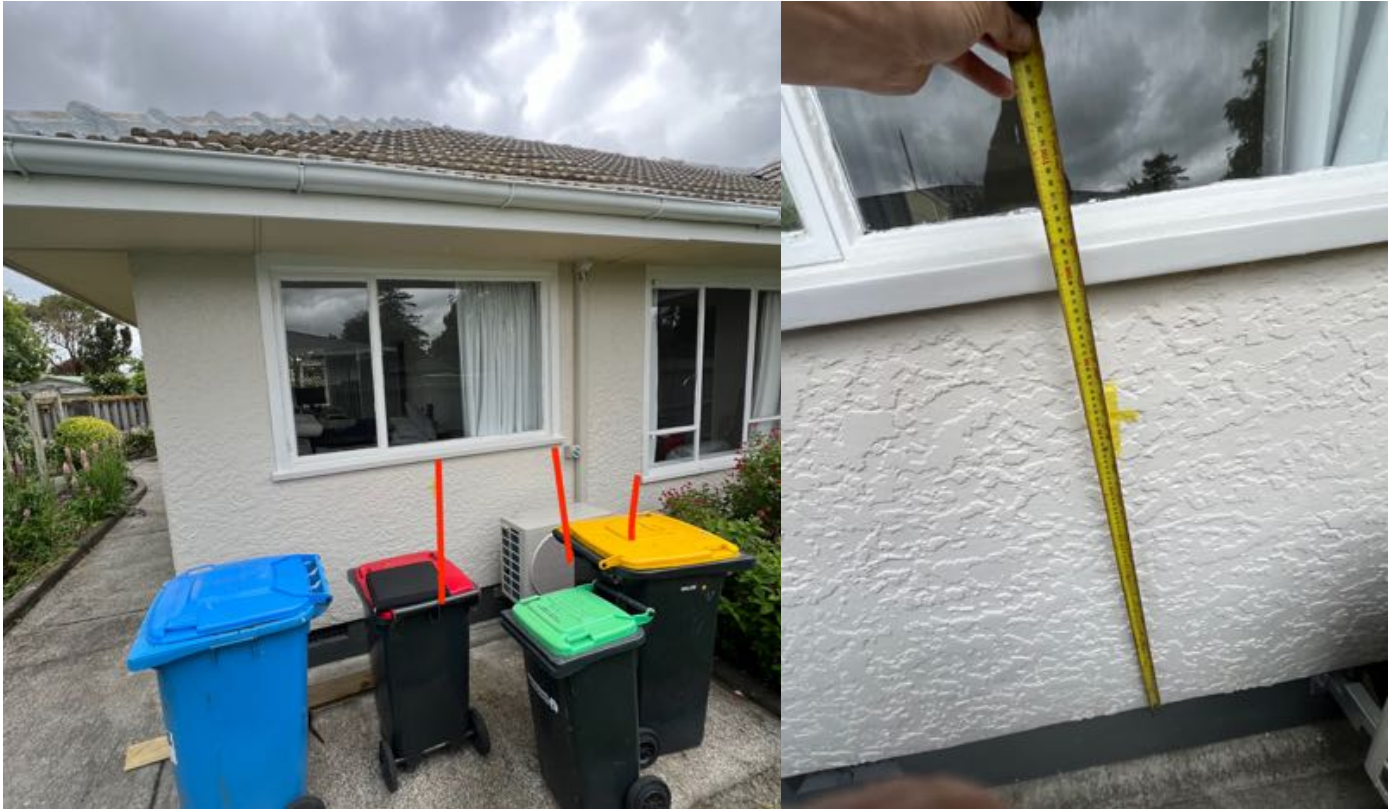
Figure 3 & 4: West elevation. Signs of cracking in Stucco.
