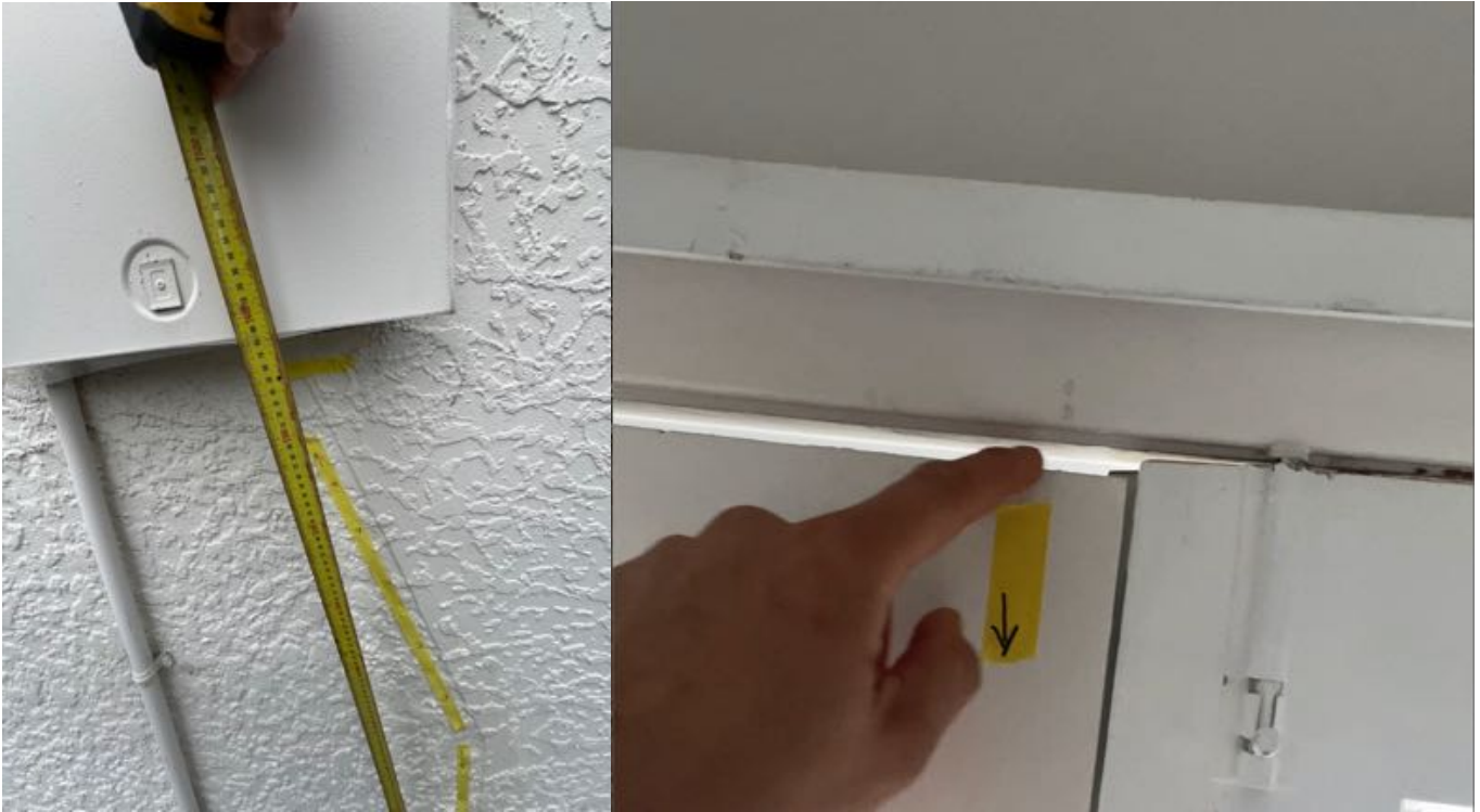
Figure 15 & 16: East elevation continued (driveway). Signs of cracking in Stucco. Photo on right showing double door on East elevation (entrance). Signs of door frame dropping due to floor level
