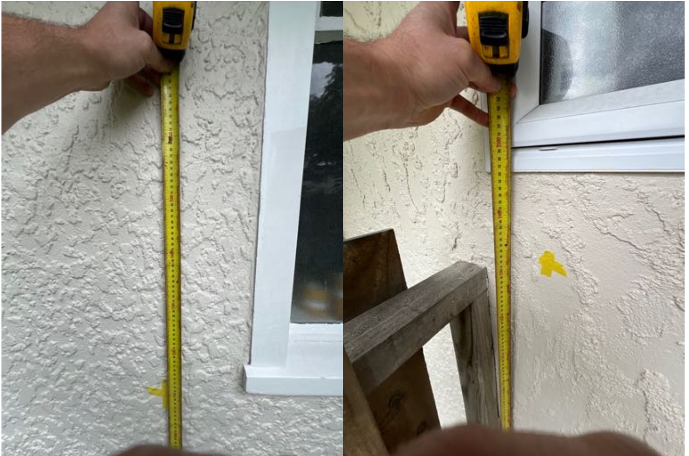
Figure 11 & 12: South elevation continued. Signs of cracking in Stucco.
