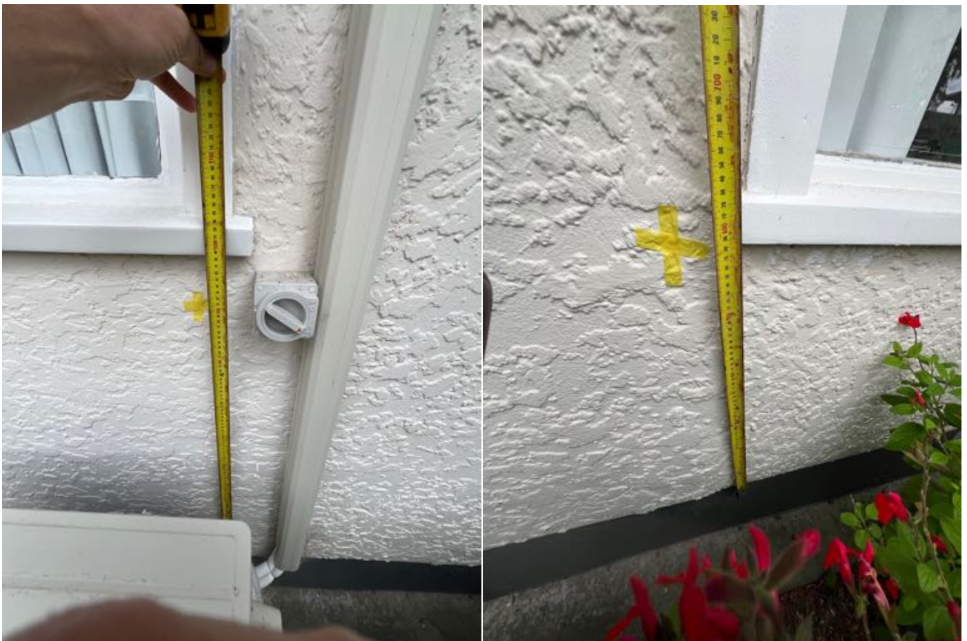
Figure 5 & 6: West elevation continued. Signs of cracking in Stucco.
